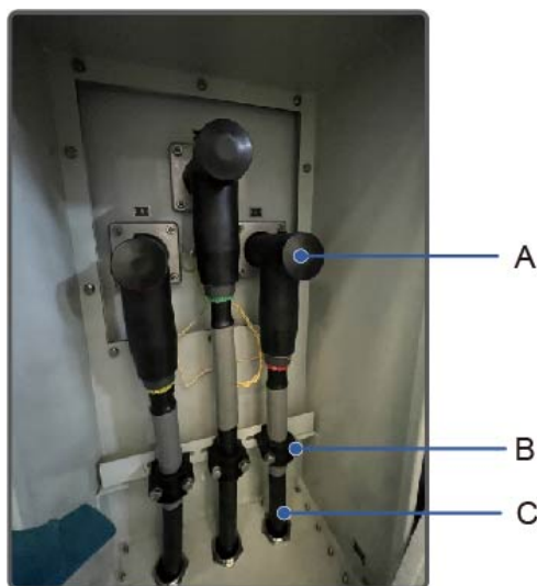
figure 6-5 Cable compartment of the transformer
